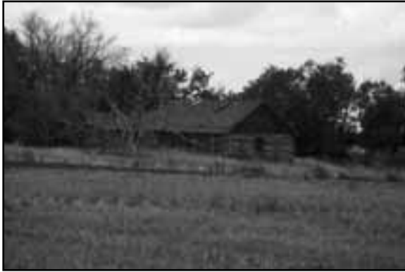
Log-constructed house, BN00-032. This is an example of a large intact ell-shaped log house. Future research is recommended; the property is abandoned and the integrity of the log construction should be evaluated.
